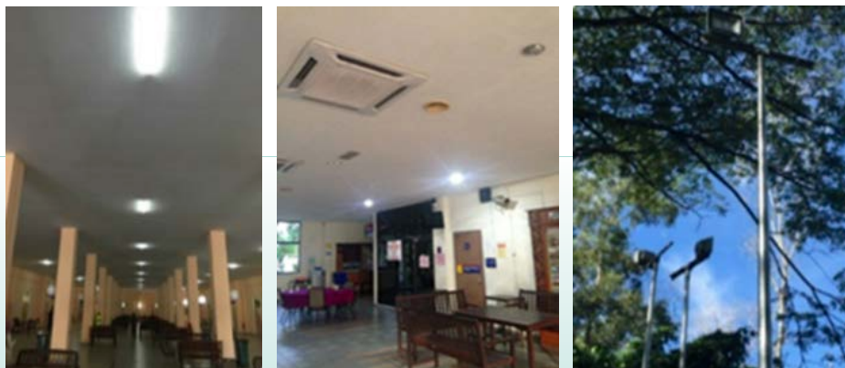
Figure 2.3: The use of energy efficient florescent and LED lights
