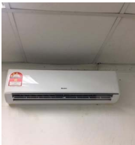
Figure 2.1: Installed 3-Star rating Split Unit air-conditioner
