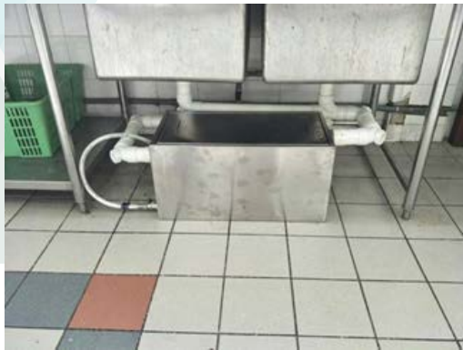
Figure 2.18: Organic oil/grease trap at eating outlets with kitchens
