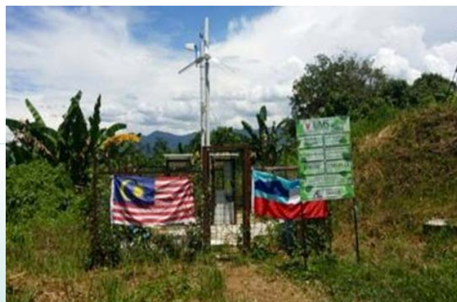
Figure 2.9: Wind turbine system on UMS Peak to supply electricity to meteorological data logger
