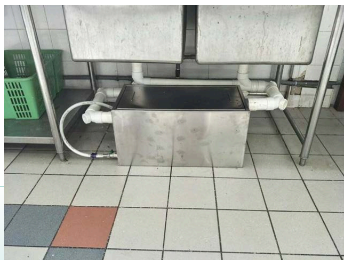
Figure 2.32: Organic oil/grease trap at eating outlets with kitchens
