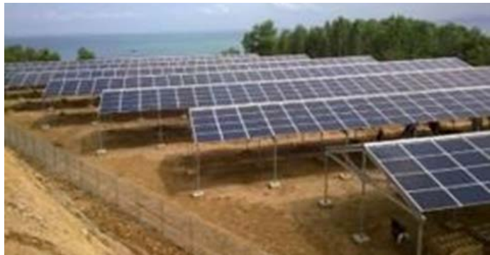
Figure 2.5: Sabah's largest solar energy generation plant located in the district of Kudat
