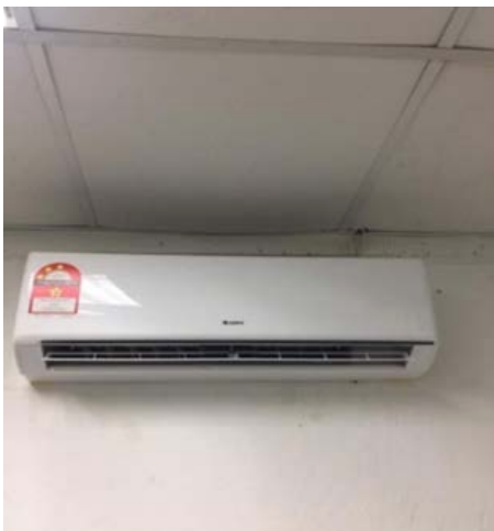
Figure 2.1: Installed 3-Star rating Split Unit air-conditioner
