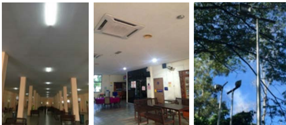
Figure 2.3: The use of energy efficient florescent and LED lights
