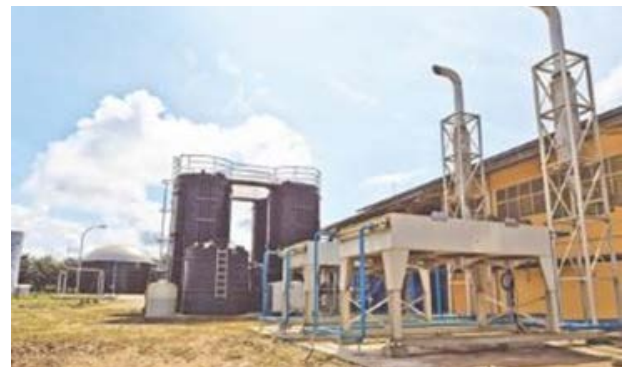
Figure 2.8: Sabah's biogas energy generation plant located in the district of Sandakan
